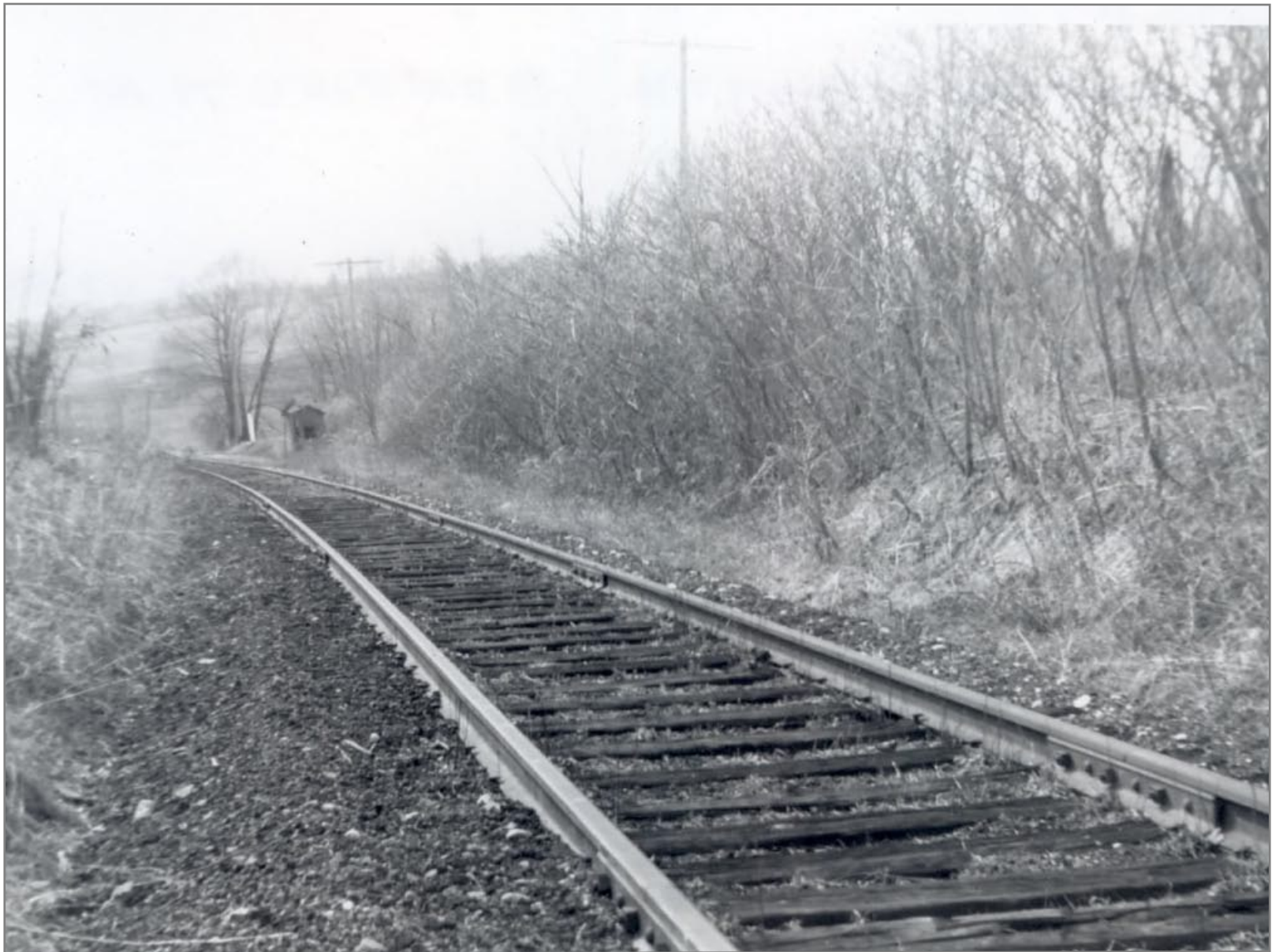
Old Siding Started For White Creek Station on Right - Tool Shed in Background Looking West 4/15/1962
