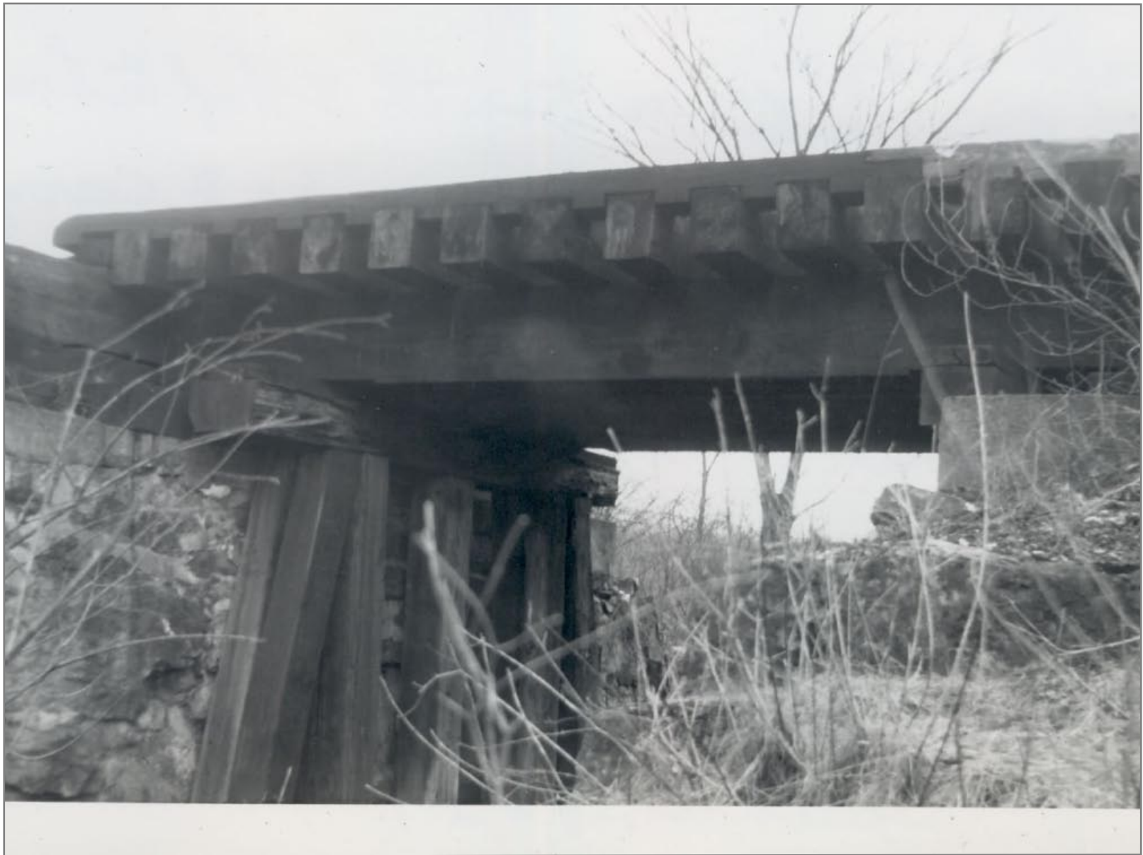
Small Bridge Between 1st and 2nd curve north of North Bennington 4/21/1962 Bridge Cribbing Installed to Support 90 Class Locomotives
