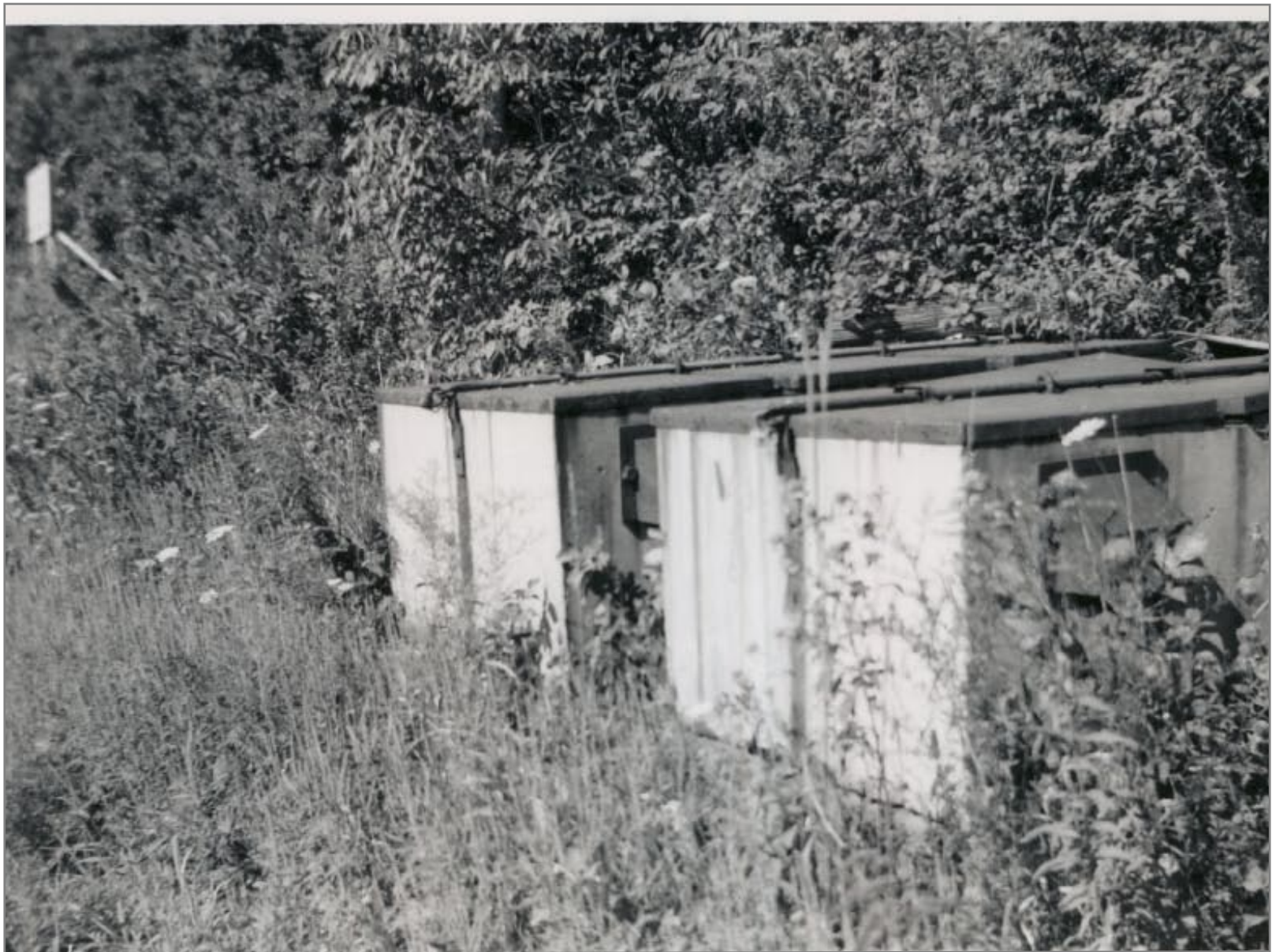
Chatham Branch Battery Boxes for Crossing Signals on Route 7 near Bennington 8/1960
